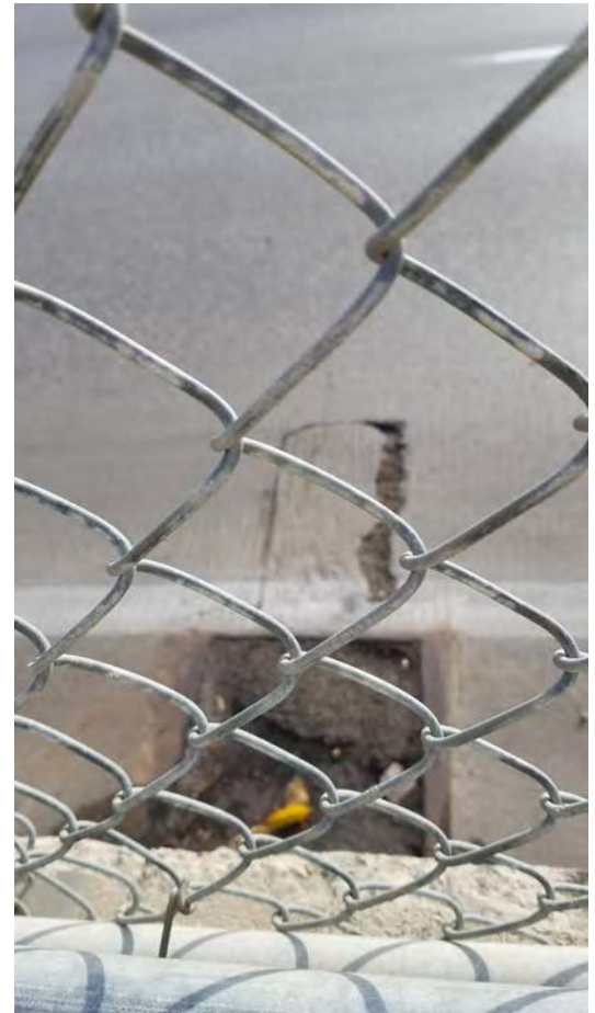
Figure 11 - Failed patch over abandoned deck drain west barrier (north drain)
