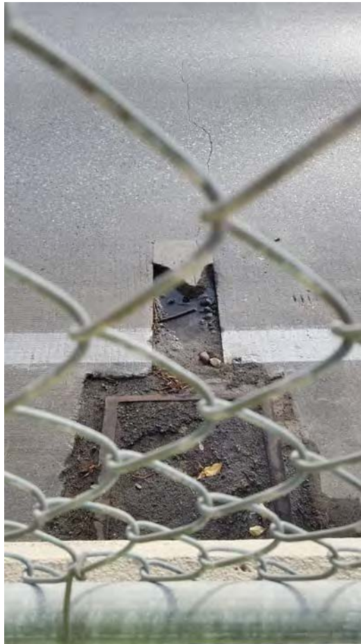
Figure 10 - Failed patch over abandoned deck drain along west barrier (south drain)
