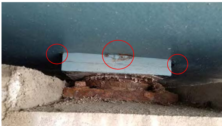
Figure 7 - Bearing at North Abutment. Girder No. 4 Note notch cut into top of pedestal because pedestal was cast too tall. Also note failed paint coating in vicinity of welds between sole plate and girder flange.
