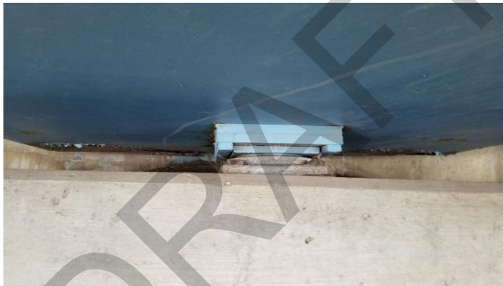
Figure 9 – Bearing at North Abutment under Girder No. 2. Note bars on sides of sole plate that provide lateral restraint.
